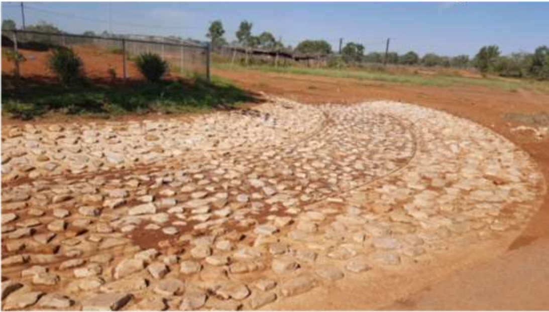
21 – Stone pitching drain protection at the bottom of Rainbow Street has been cleaned
