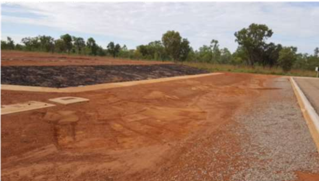
10 – Scouring on road 4 on Lot 511 batter fixed
