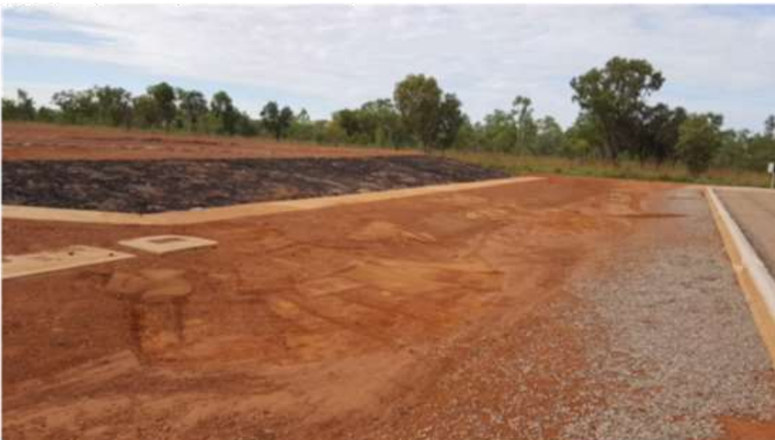
10 – Scouring on road 4 on Lot 511 batter fixed
